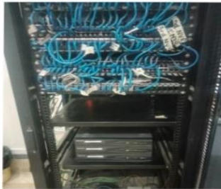
PSK Server Rack Maintenance & Tagging
