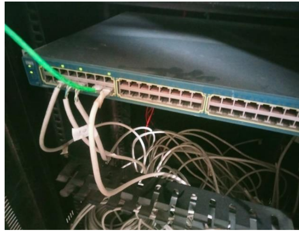
Thatta Computer Lab Network Switch Operational
